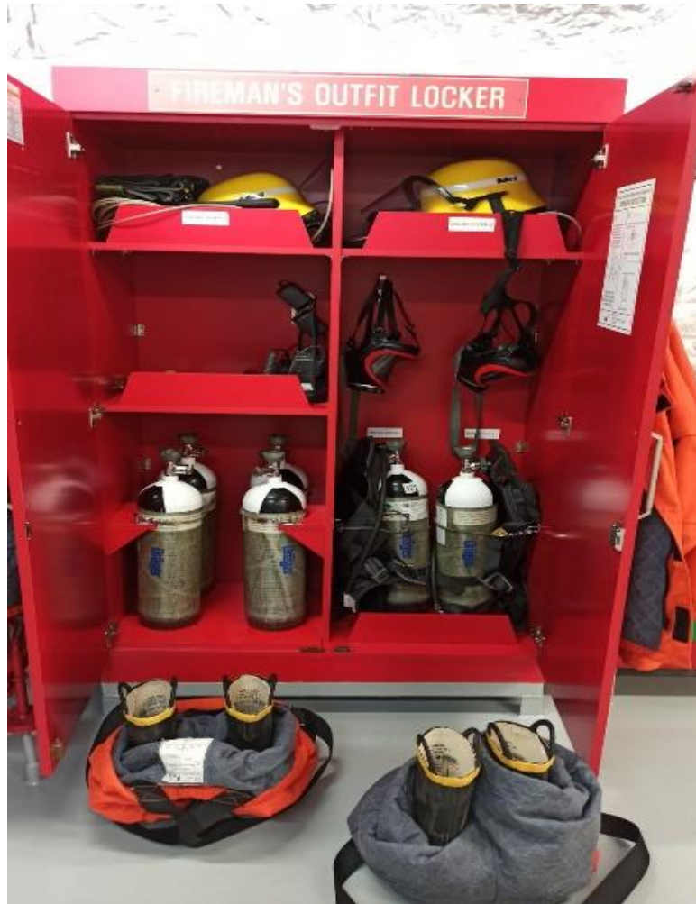
Figure 1. Fireman outfit on board (VLCC tanker)
