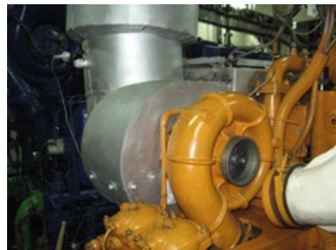
Figure 3. NAPIER C-045/C radial-flow turbocharger on SULZER auxiliary engine type 6AL20/24
