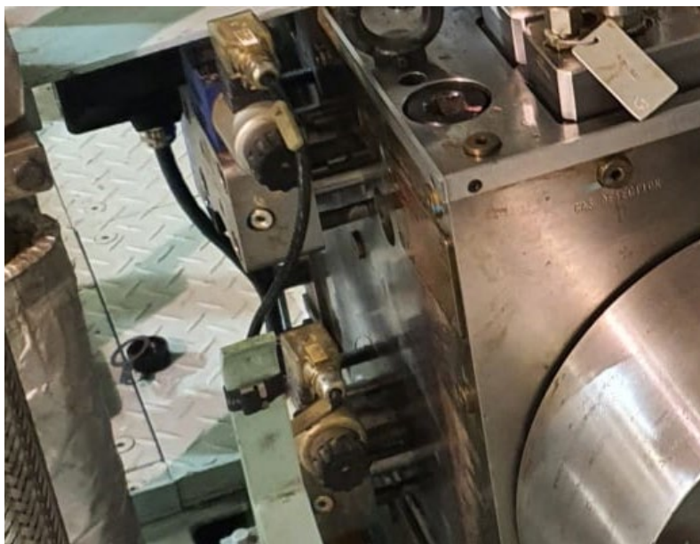
Figure 9. Blow-off valve and Purge valve (Source: Authors, 2023)
