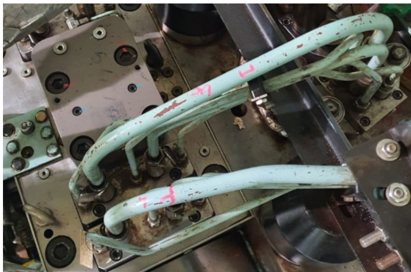
Figure 13. Five the control pipes (Source: Authors, 2023)
