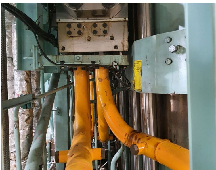
Figure 3. Fuel gas pipes (Source: Authors, 2023)
